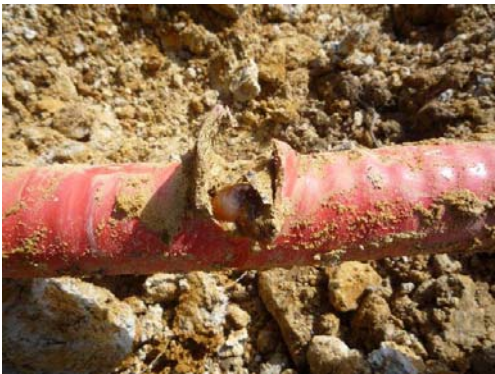
Damage to insulation cable by tent peg or spike
